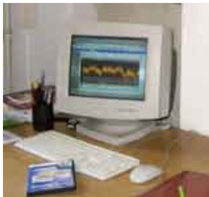
Energy2120 installed at the A. Fontana ham factory. Continuous monitoring, logging and processing of the data using the PVENGMBLDO supervisor software module
