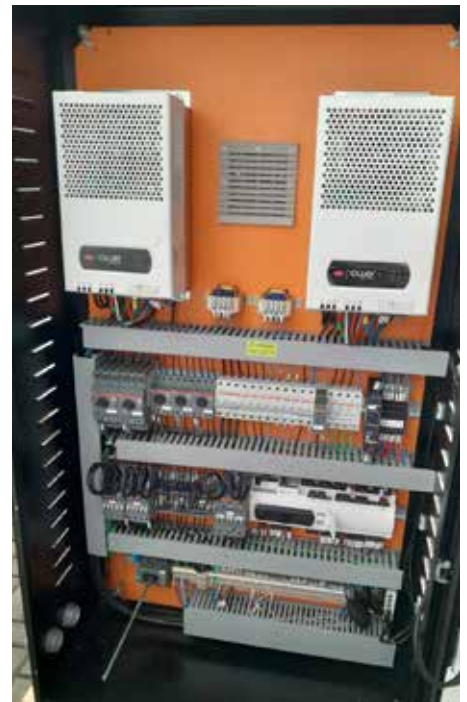
Fig. 1.b - DEMETRA unit switch board panel integrating CAREL c.pCO controller and Power+ inverters
