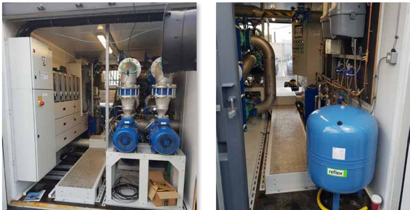
Fig. 1.c - Detail of inside the heating/cooling equipment room
