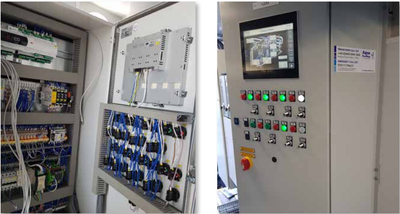
Fig. 1.b - Detail of the electrical panel with system managed by the c.pCO controller
